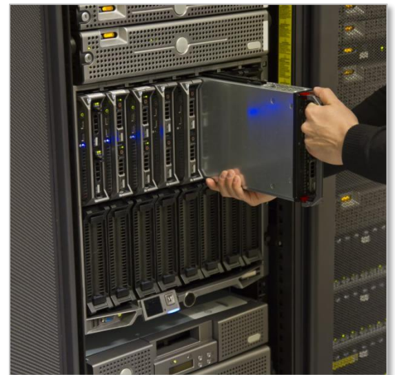
Data Center Racks
